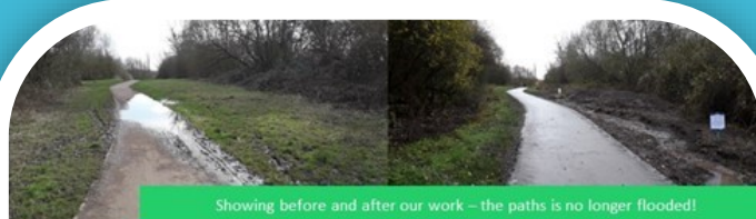
Showing before and after our work – the paths is no longer flooded!
